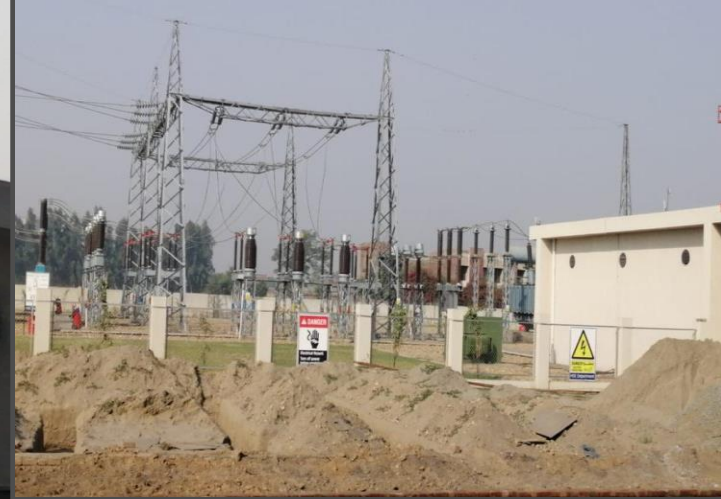
132 KV Grid Station
